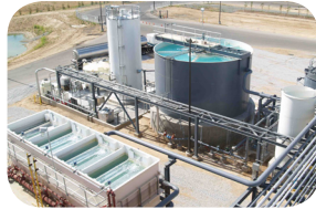
1st Zero Liquid Discharge Facility Case Study: ZLD
